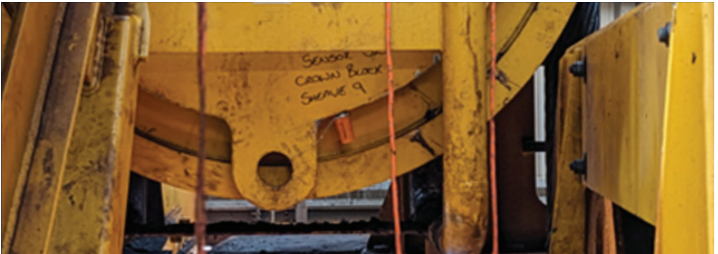
The West Neptune's main well crown block sheave is complete with the driller's side sheave sensor visible. Seadrill can monitor vibration and RPM of the sheaves, assessing their condition and remaining life for continuous, disruption-free operations.
